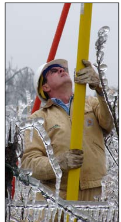
Jerry Cochran, Heartland, works on the ice-coated lines.
