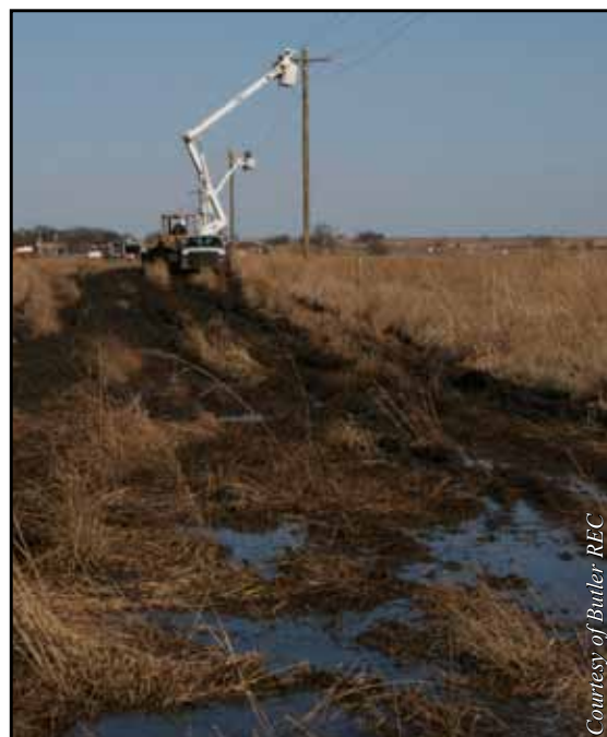
Winter weather quickly warmed, leaving roads muddy and impassable. Equipment was brought in to drag the line trucks to the damaged areas.
