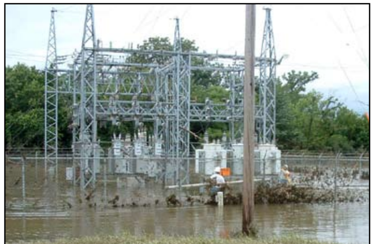
Radiant line crews begin cleaning the substation of tree limbs and other debris in the standing water while repairs begin.
